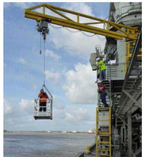
Barge Access System with Powered Trolley
