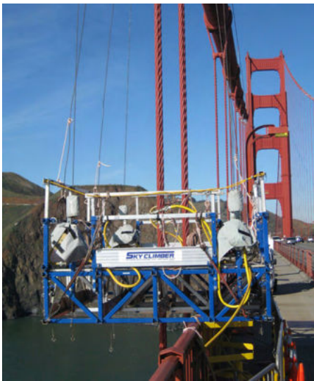
Bridge Cable Maintenance Platform
